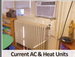
Current AC & Heat Units
